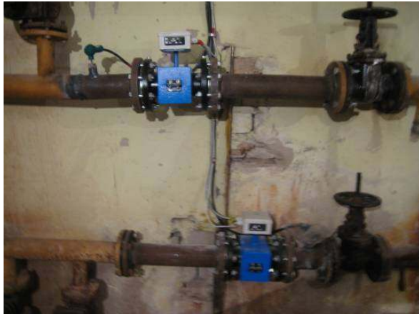
Meter for heating
