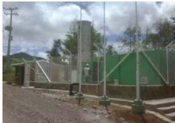
Landfill-based biogas collection and flaring. Pasto, Colombia
